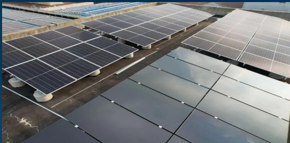
2024: Rooftop Solar Project, Jiangsu Province
