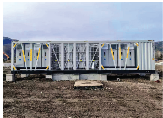
100MW / 200MWh BESS project supplied by Kehua in Bulgaria
