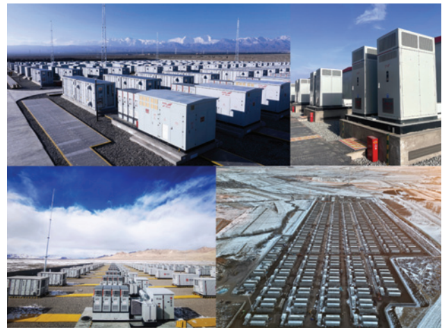
Grid-forming BESS projects supplied by Kehua across Northern China
