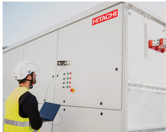
Hitachi Energy PCS unit at a customer site.
