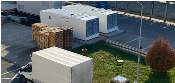
Diesel Generators for last instance usage
