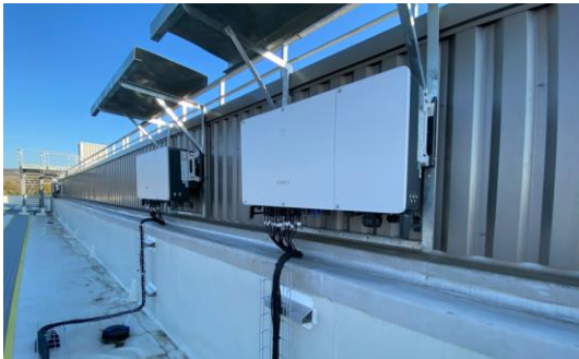
Solar PV Inverters
