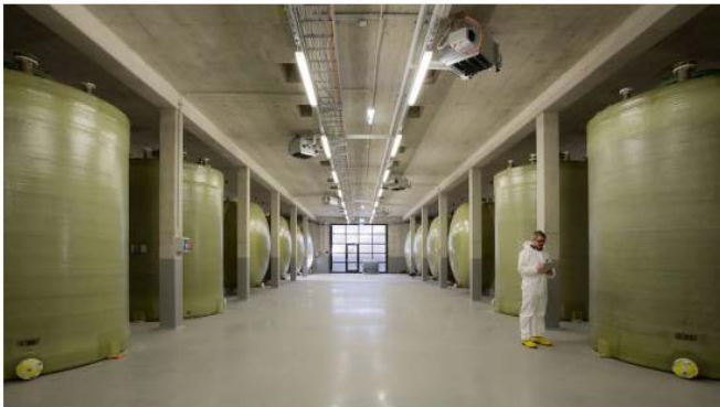
Liquid electrolyte tanks at a large-scale vanadium flow battery demonstration and research project. Image: Fraunhofer ICT.
