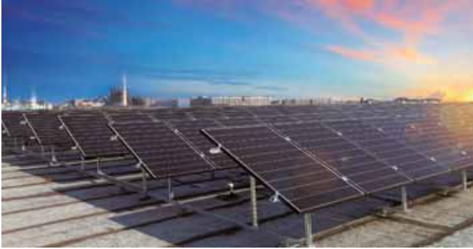
Largest Global Rooftop Project Using Shingled-Cell Modules Changzhou, China | 1.5MW
